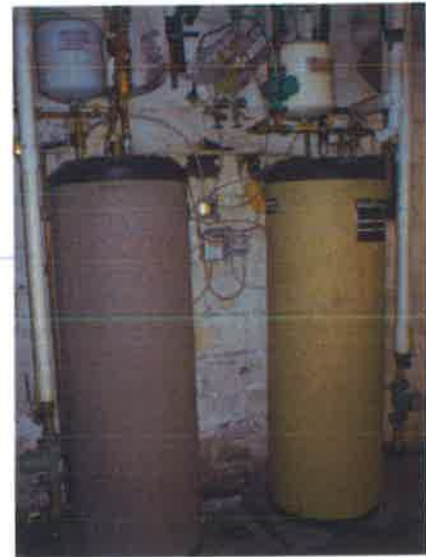
OIC Domestic Hot Water
