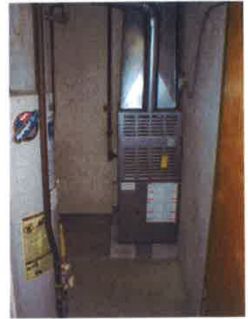
Apartment Mechanical Closet
