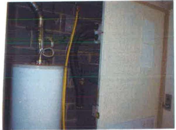
Apartment Mechanical Closet
