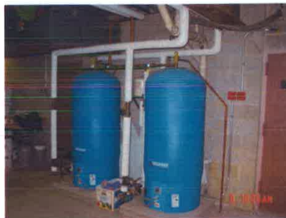
Hot Water System
