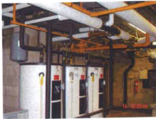
Central Hot Water
