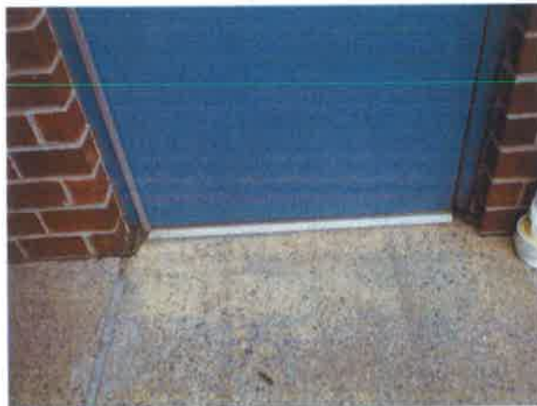
Rusting Exterior Doorframe
